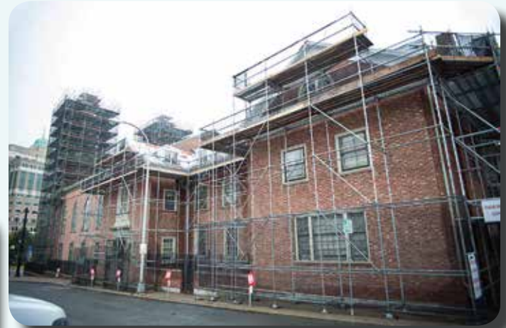
Side view of First Church renovation showing multiple roof elevations and working platforms. Renovation is estimated for completion in November 2015.
