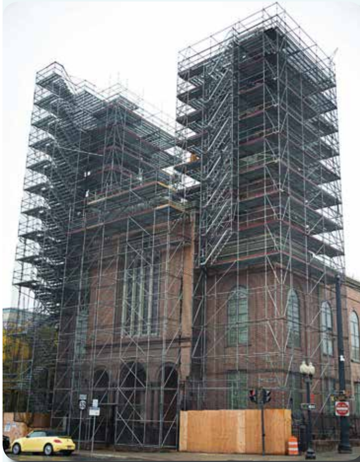
Front view of First Church renovation in Albany, NY. Tri-City installed 11 working levels of Layher Allround Scaffolding to provide access to multiple roof elevations, chimneys, and two spires in addition to overhead protection of sidewalks and doorways.
