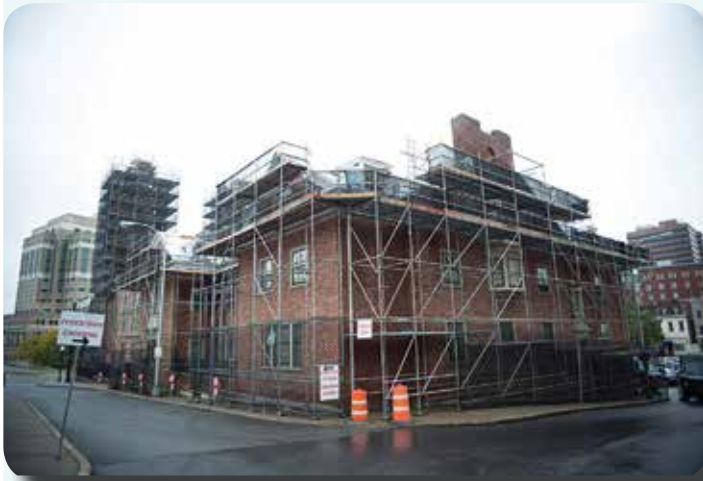
First Church renovation from behind church building. Layher Allround system scaffolding overcame ground elevation changes pictured through built-in versatility.
